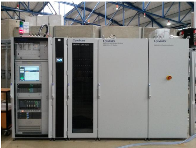
Figure 1: Radiofrequency amplifier delivering 75 kW RF power for the storage ring DELTA.
